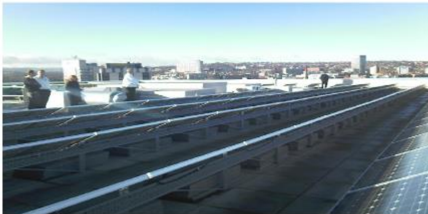
Rooftop PV Panel Array
